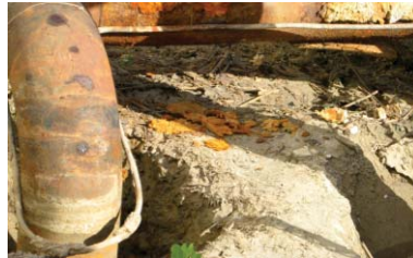
Real life problem 2 Corrosion of Piping
